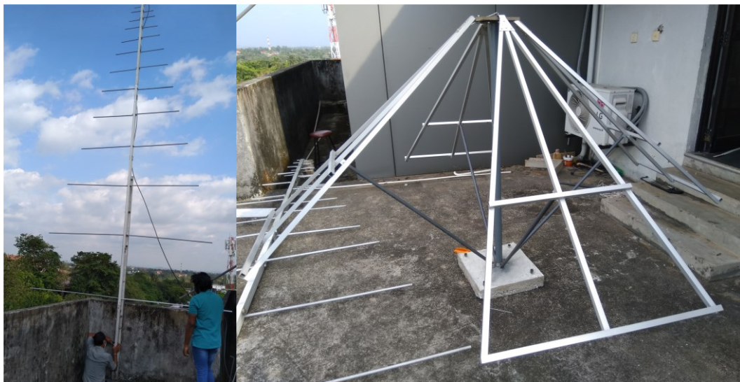
Figure 6: Left: 6 m tall Log-Periodic antenna of the existing CALLISTO receiver. Right: The construction of Long Wave antenna for the proposed polarization measurements of solar radio bursts.
